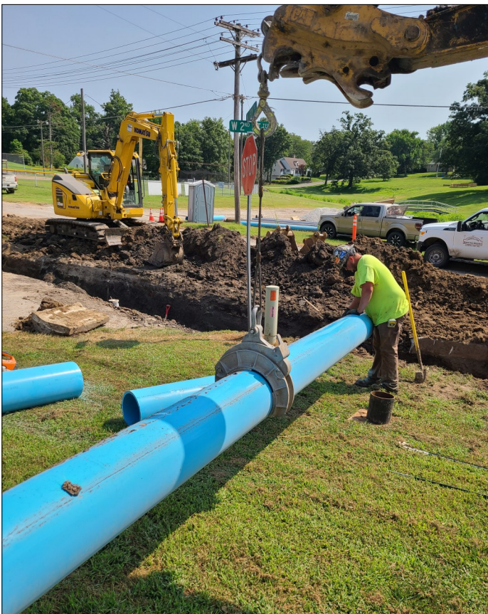
A contractor readies a 12-inch water main for installation, part of Carrollton's major water system overhaul.
