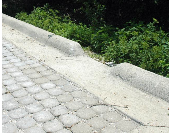
Figure 64-A: Example of a break in a continuous curb to provide for stormwater flow.
