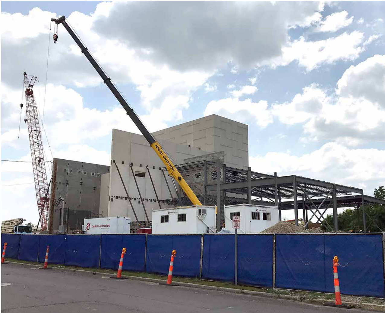
Construction on the Kirkwood Performing Arts Center is moving along. This section, as seen from the construction yard, is where the stage and "house" areas will be. Work is now being completed on the interior foundation walls, which must be completed before the house area can be enclosed.
