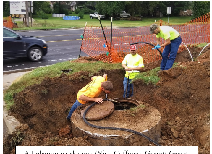
A Lebanon work crew (Nick Coffman, Garrett Grant, and Tyler Wasmer) install a pressure main into a manhole. (photo: City of Lebanon)
