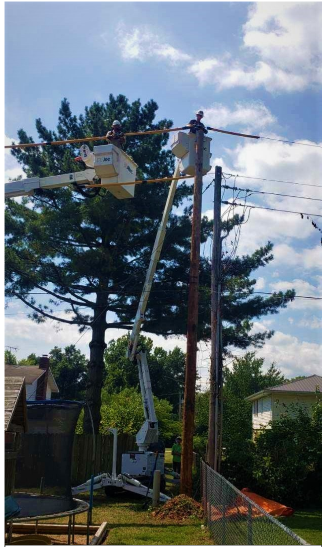
Lebanon lineworkers Matt Crump, Andrew Bowman, and Steven Vickers replace a distribution pole. (photo: City of Lebanon)
